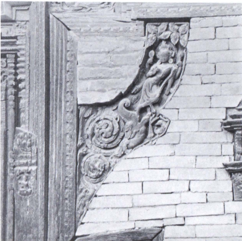
b) Patan, Nārāyaṇa temple, portal on south side, detail, missing parts replaced with brickwork
